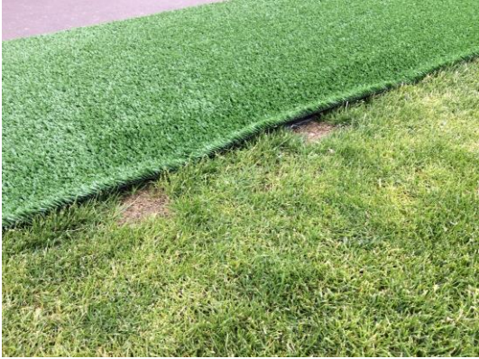
Poor interface between natural and artificial turf at the perimeter of a pitch – a major trip hazard and likely to cause player injury.
